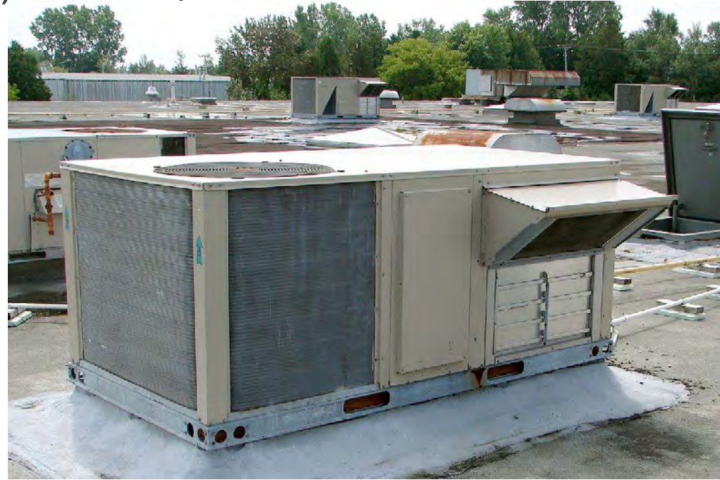
Heat Pump Rooftop Package Units
