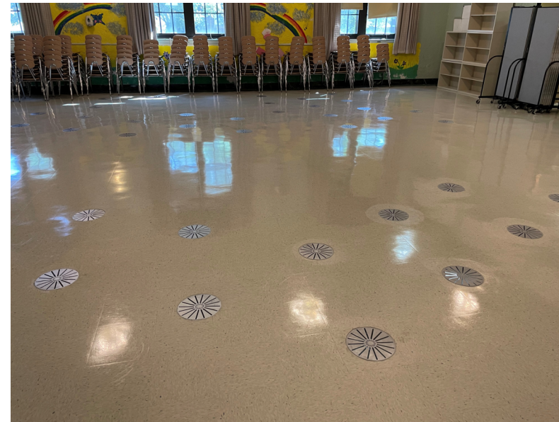
AUDITORIUM FLOOR DISPLACEMENT DIFFUSERS
