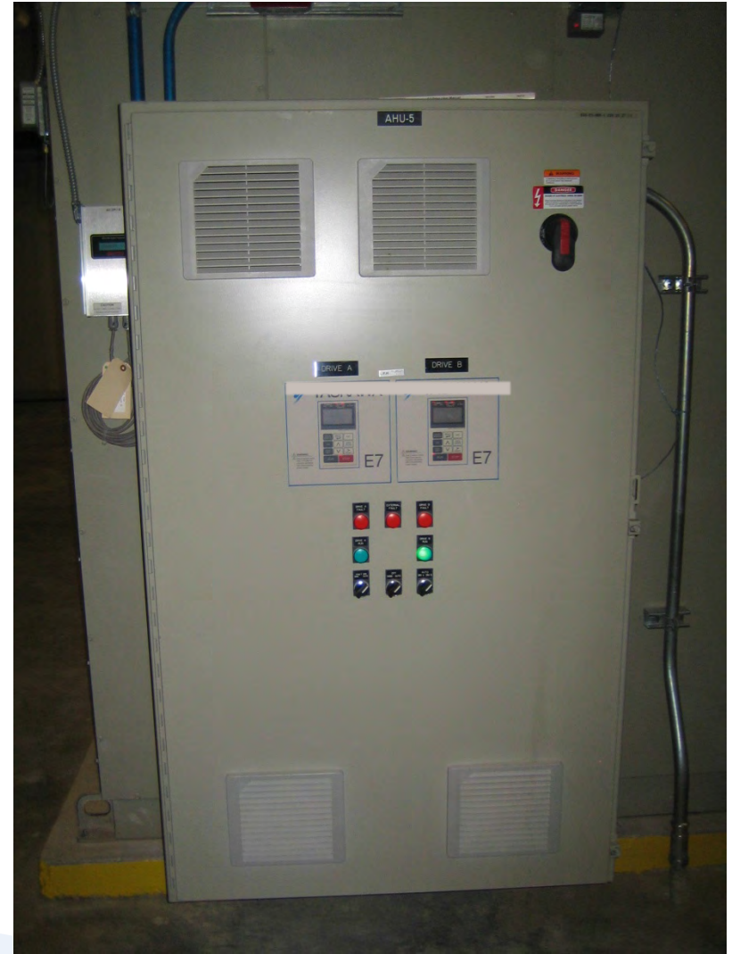
Dual VFD without Bypass
