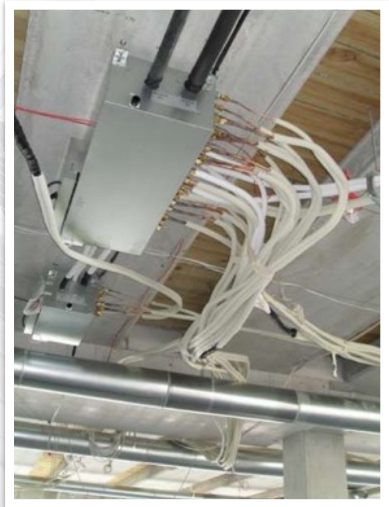
Examples of Poor Installations
